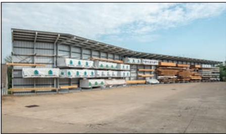
2016 New Racking for Lumber Storage
